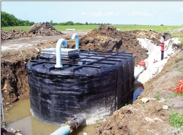
The Paola/RWD 2 interconnect vault above is located north of Paola and just north of the new Paola storage tank on the road to Miami RWD 2's water treatment plant. The vault is nearing completion and the interconnection function should be online later this summer.
