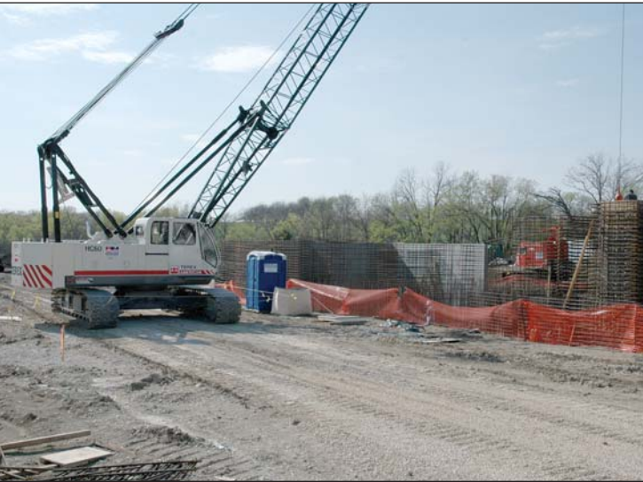
Work progresses at the PUA water treatment plant site on the Marais des Cygnes River south of Paola. Manhattan, Kansas based Walters Morgan Construction, Inc., employees work with the company’s new crane to ready forms for concrete on the new plant building. The plant is targeted for completion sometime in late 2009.
